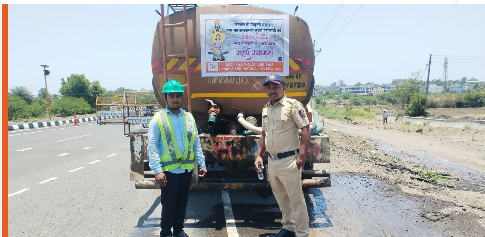
4320- Shirdi Sinnar Road Project Sprinkling of water on the road to combat heat and making it easy to walk for barefoot pilgrims.
